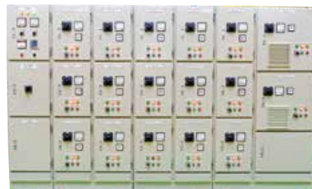
Motor Control Center (MCC)
