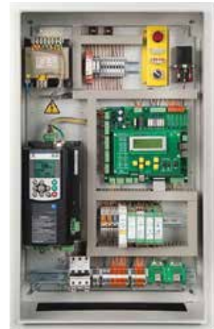
Elevator Control Panel
